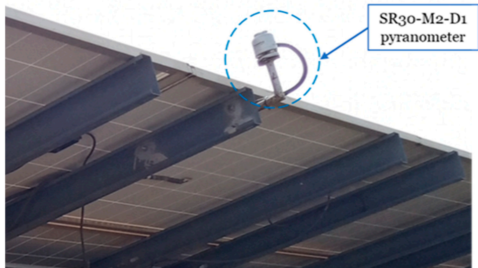
Figure 7. Weather Station in the PV array site.
