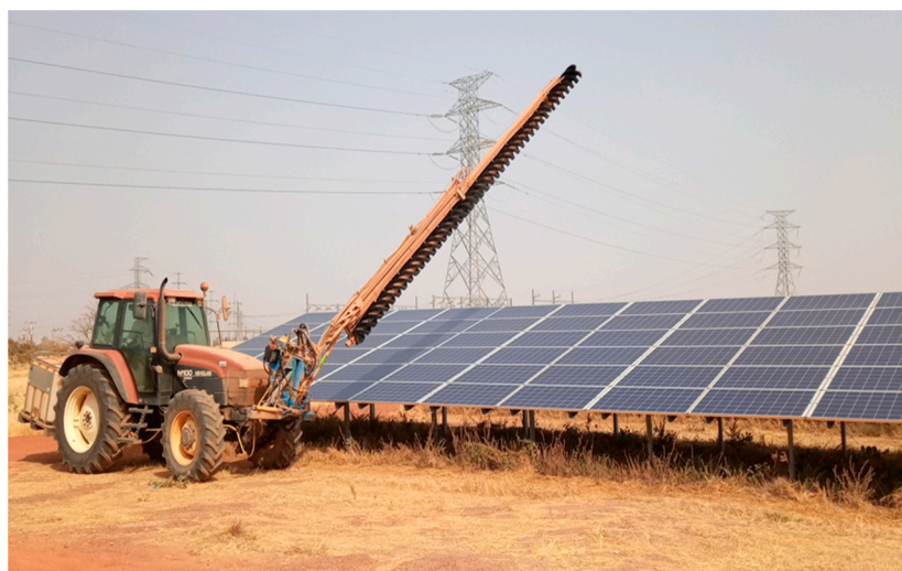
Figure 5. Zagtouli PV Plant semi-automatic cleaning System.
